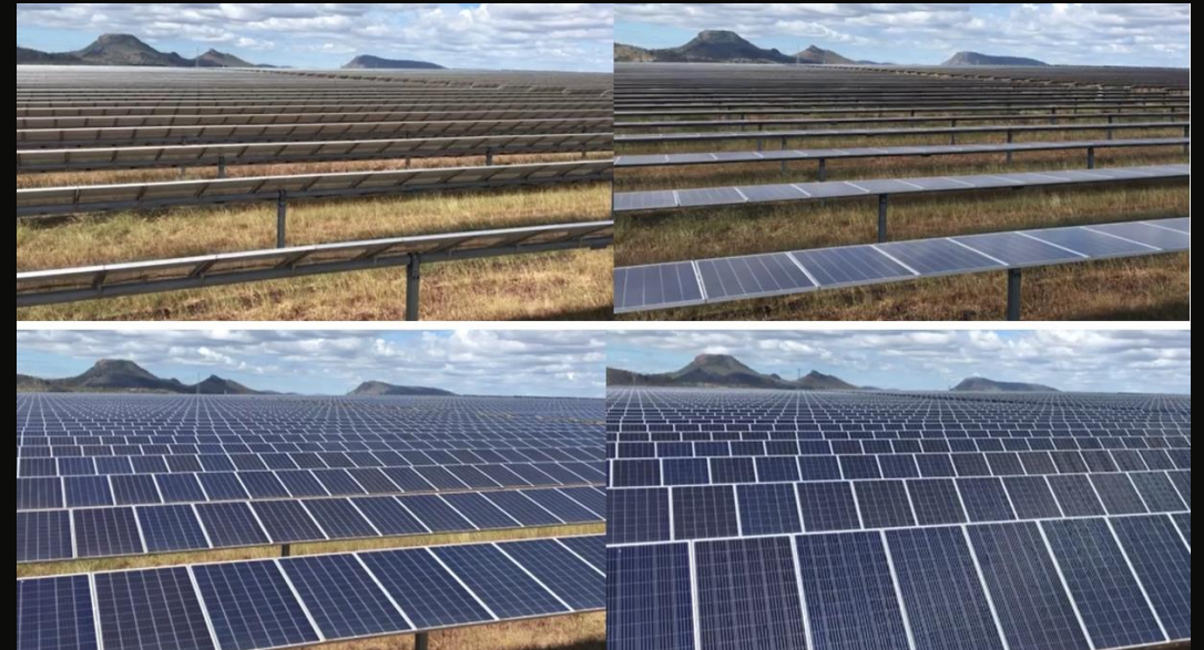
East-west single axis tracker system, finished array (Note example is in Australia).
